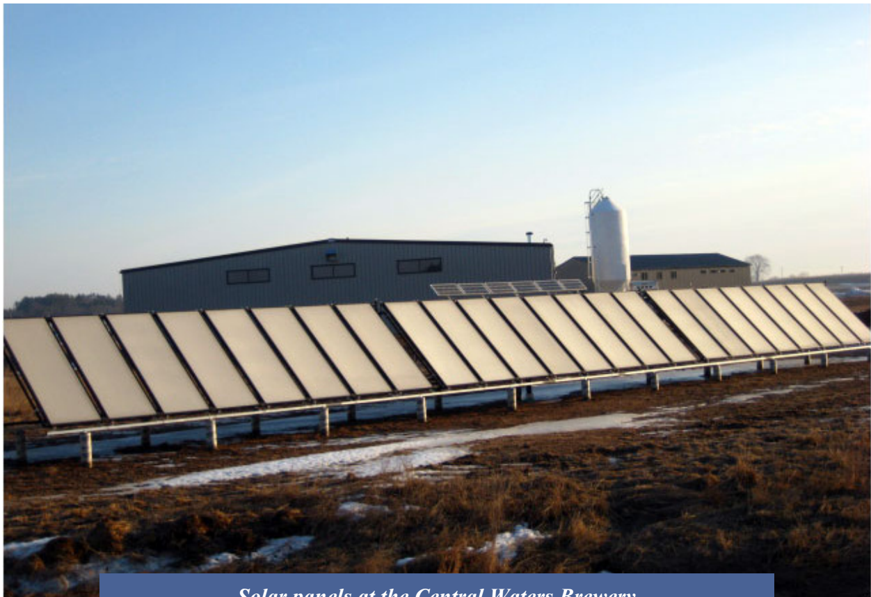
Solar panels at the Central Waters Brewery
