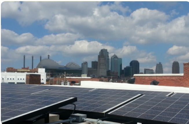
One of many solar roof projects in Kansas City's urban core.
