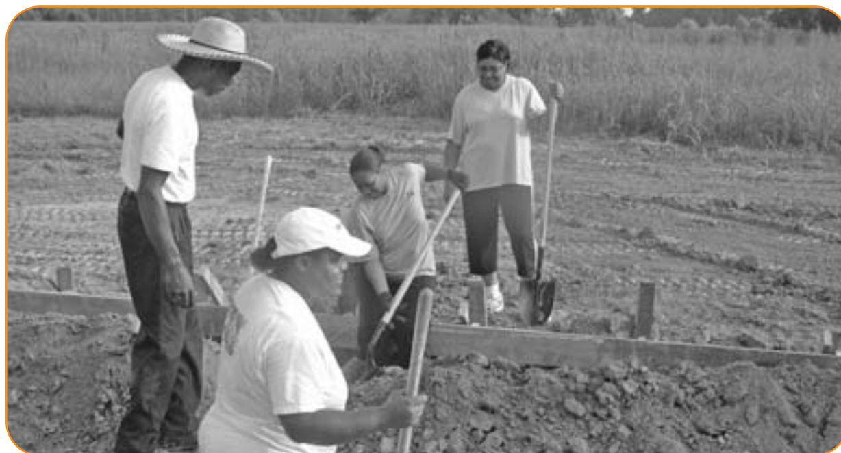
Future neighbors work together to help build their homes under Esther Stewart Buford Foundation's mutual self-help program in Yazoo City, Miss.
