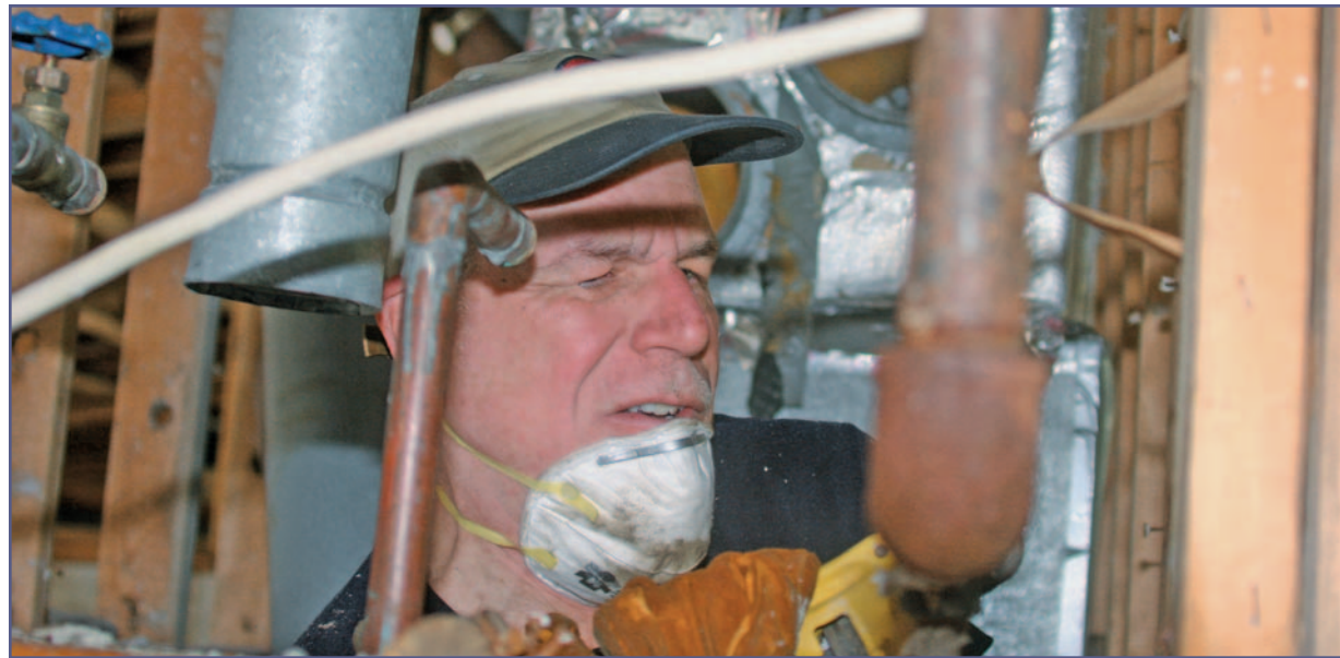
Below: A volunteer removes plumbing in a church rectory submerged by Katrina.
