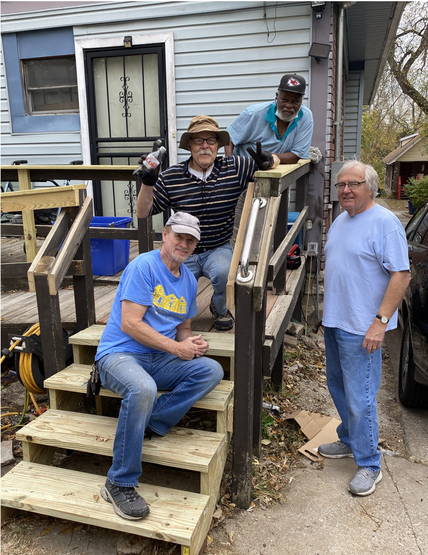
Photo of the Volunteers Repairing a Porch. Courtesy of Front Porch Alliance.
