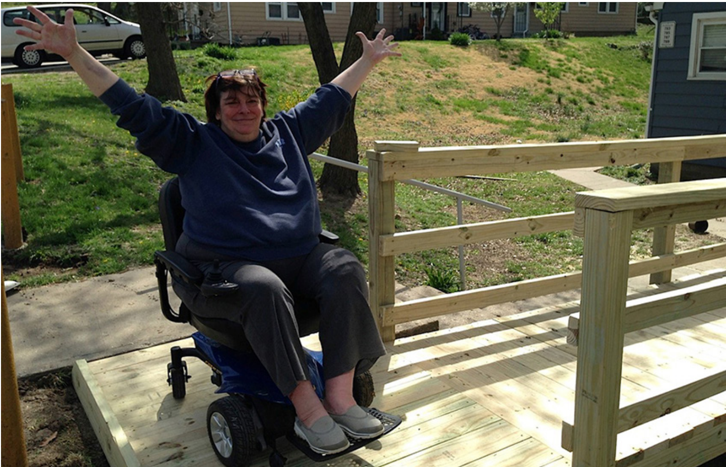
Photo of HopeBUILDERS volunteers installing a new ramp and a happy resident. Courtesy of HopeBUILDERS
