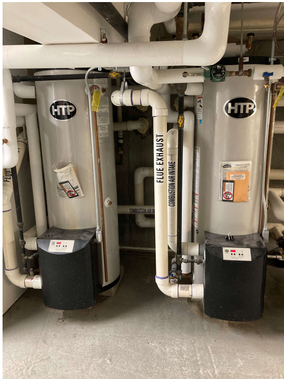
Domestic Hot Water 2 80 gallon gas fired tanks.
