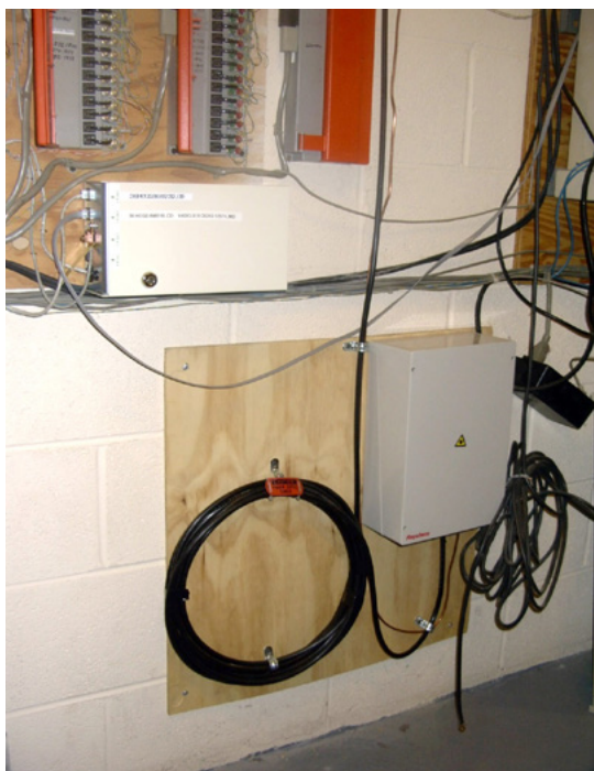
Figure 7: Wall-mounted fiber termination cabinet
