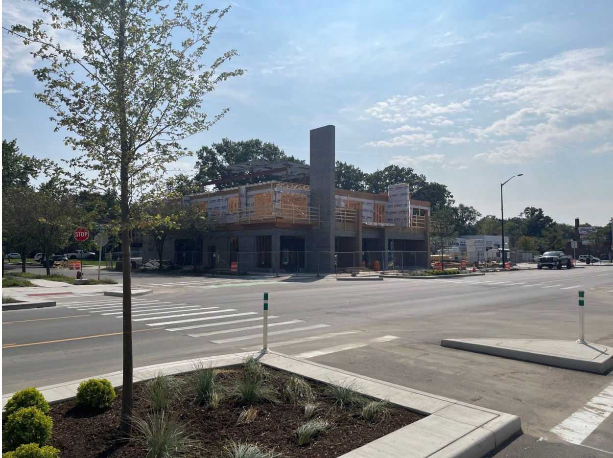
Work in progress at The Ribbon in East English Village. COURTESY OF JPMORGAN CHASE
